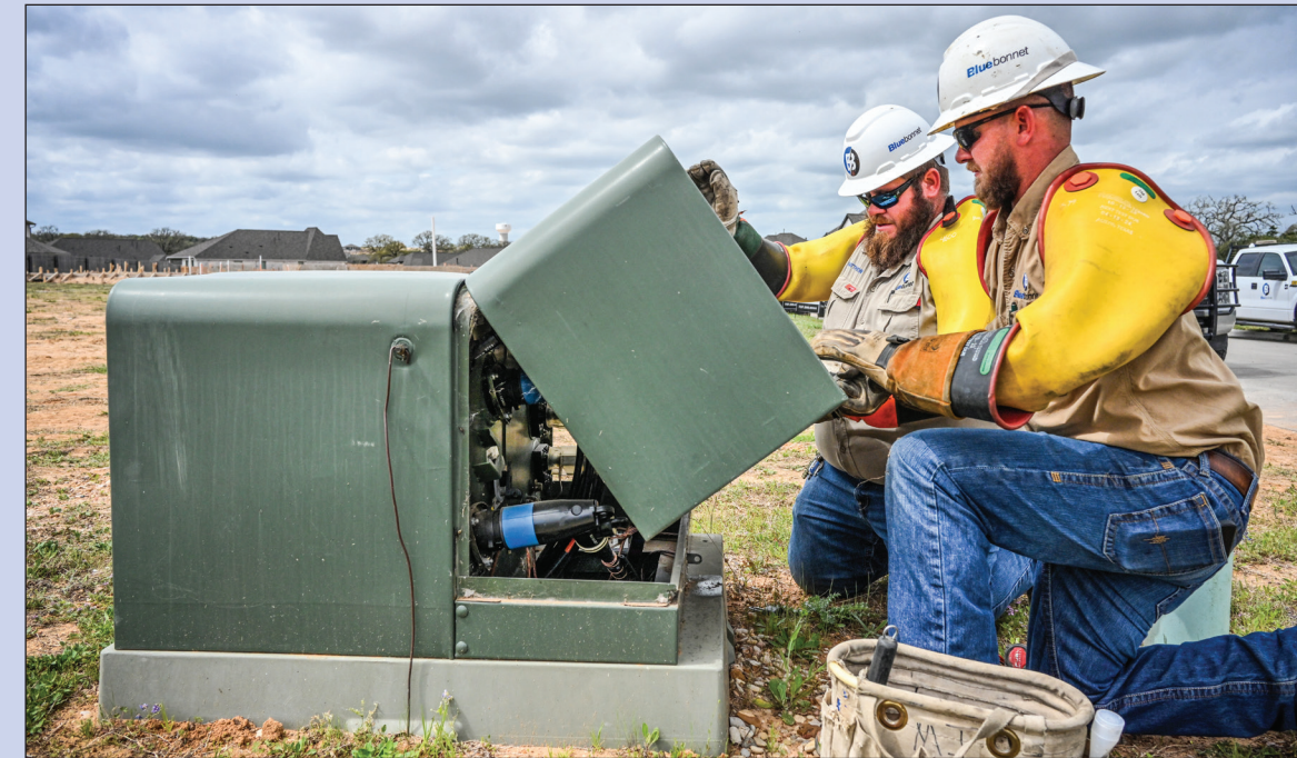
Bluebonnet journeymen Matthew Jones and Matt Mole, from Maxwell, open an underground transformer in The Colony subdivision in Bastrop to upgrade the equipment. Bluebonnet is constantly upgrading its system to provide safe, reliable power.
