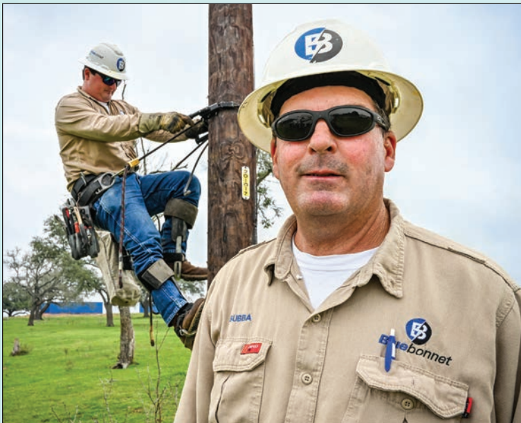
At left, Trey Townsend descends a pole behind his father, Bubba, at a new construction site in Red Rock. Read more about them on Page 18 .
